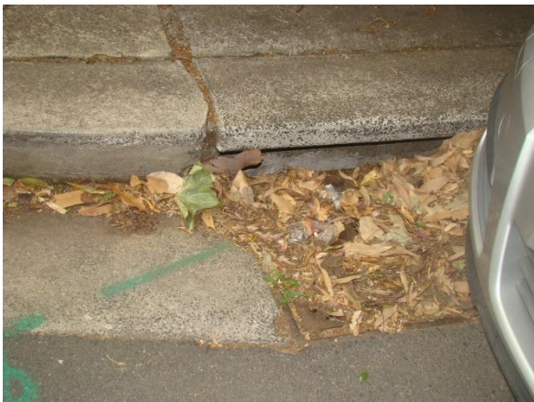
Figure 28. Street gutter inlet along Mitchell Lane – obscured by dry foliage, looking east.
